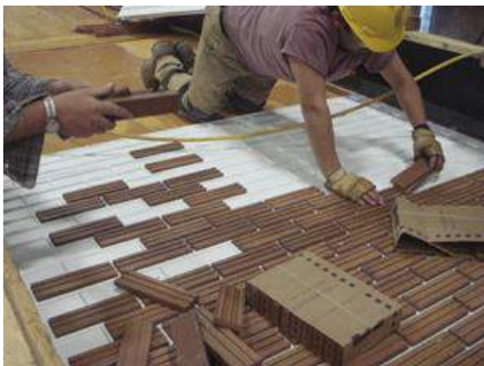
Figure 6.5: Installation of thin brick under a controlled environment. Image courtesy of Scott System
